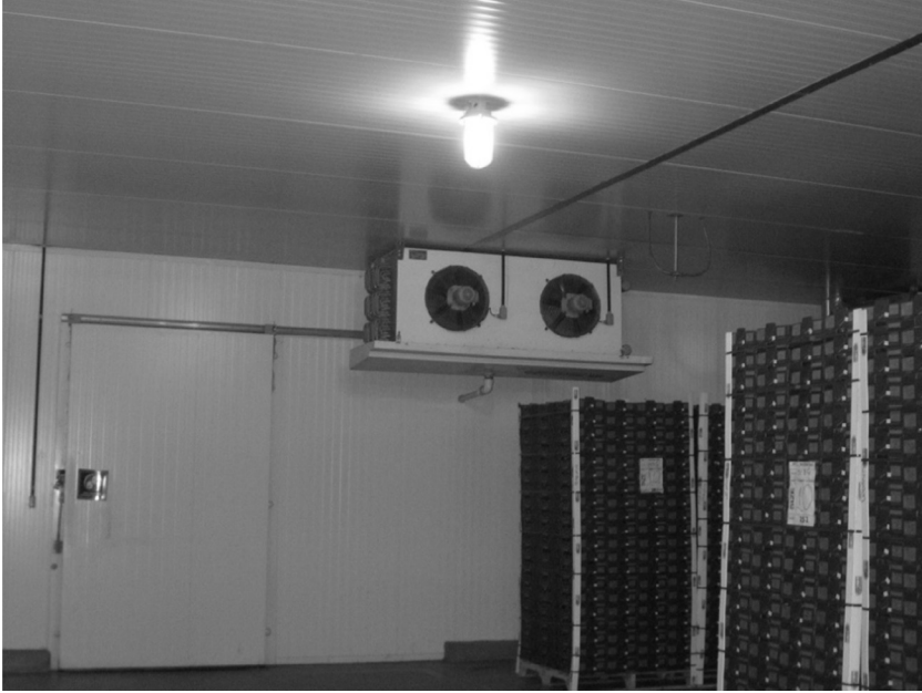
Figure 10. Cooled and palletized mangos in refrigerated storage.
